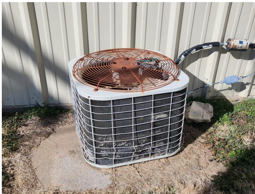
Existing A/C Unit
